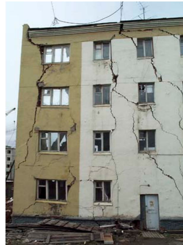
Permafrost thawing has destroyed a four-storey apartment building in Yakutia, Russia, 2001. All photos: Vladimir Romanovsky
